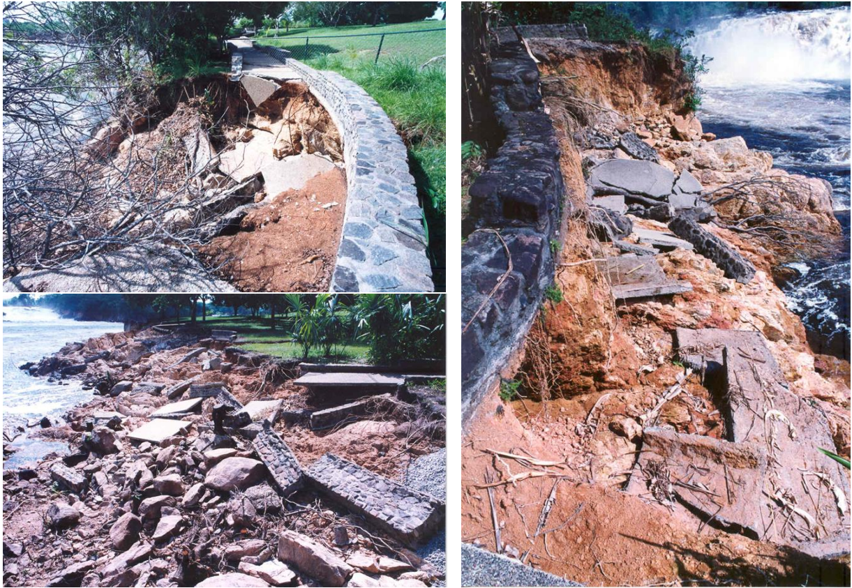
Figure B.1- 63 Extensive scour in the banks of La Llovizna Park. (EDELCA)
