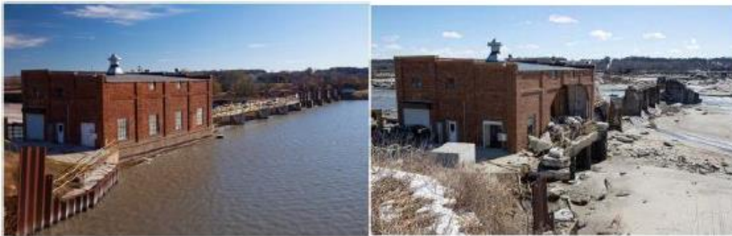
Figure B4- 10 Before and after of Spencer Dam's powerhouse failure, 2019. (ASDSO, 2020)
