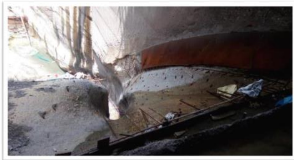
Figure B.5- 2 Shows the damages in Spillway bay no-1
