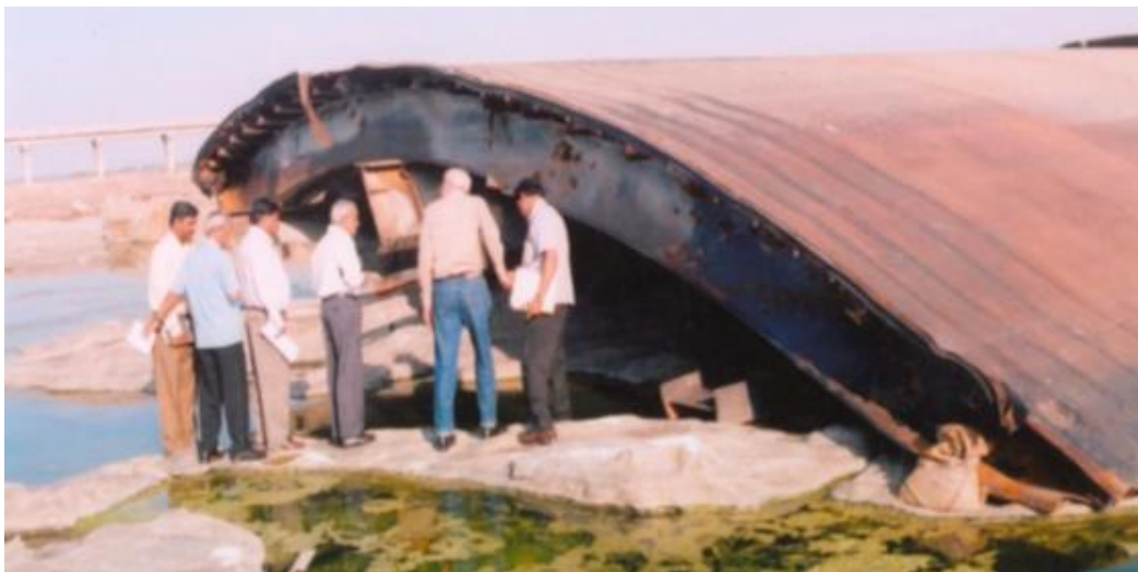
Figure B.6- 5 Damaged Skin plate of gate 5. (CWC)
