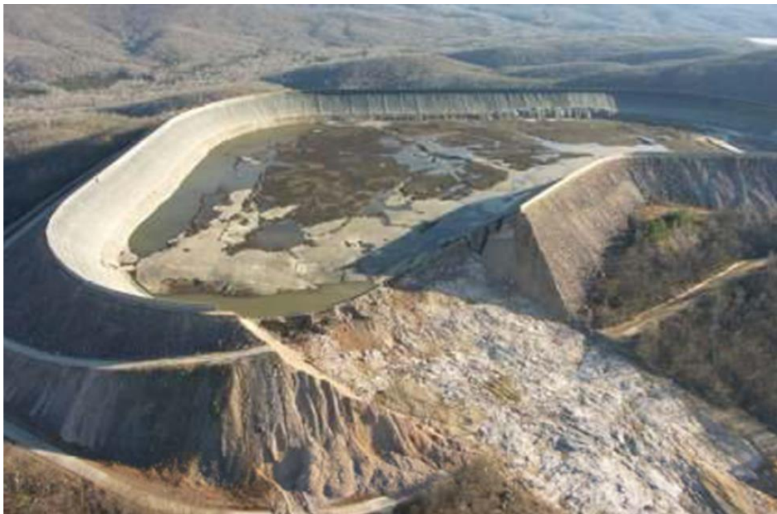
Taum Sauk Dam Overall View of the Breached Dike (Damfailures.org)
