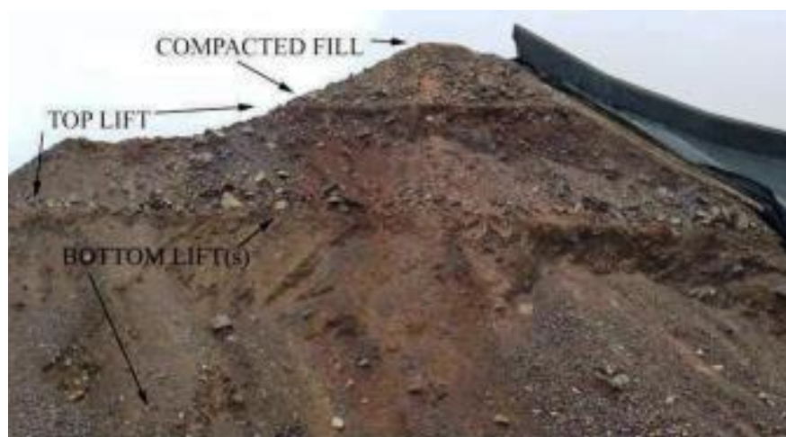
Figure B.2- 16 View of north side of breach area (FERC, 2006)
