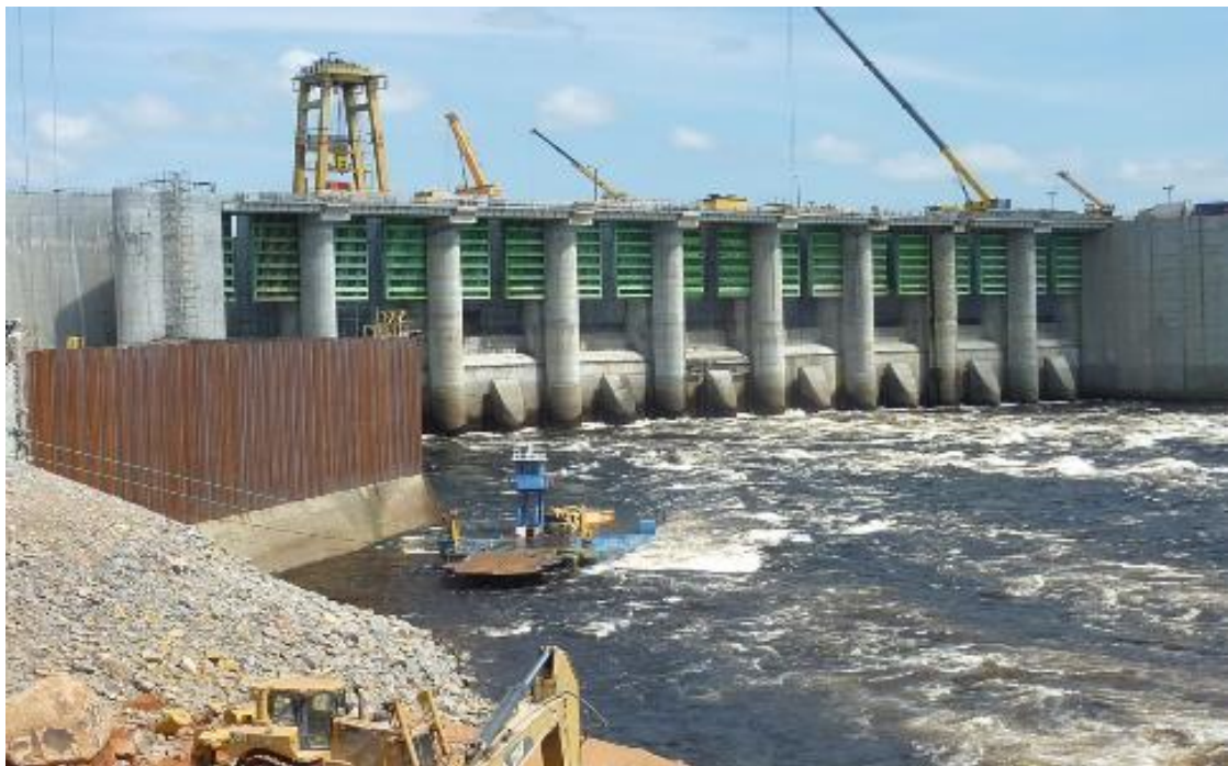
Figure C- 7 Accident with barge loaded with a truck in a dam forebay, Tocoma Project, Venezuela.
