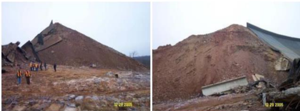
Figure B.2- 14 Left side of breach (left) and right side of breach showing layering of embankment (right)
