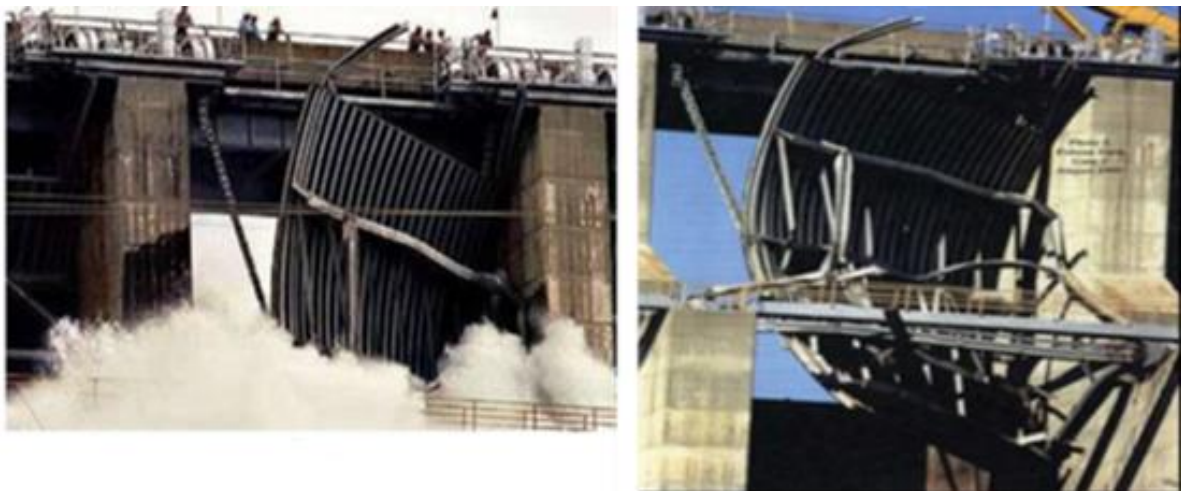
Figure E- 1 Failure of Gate of Folsom Dam, California, USA
