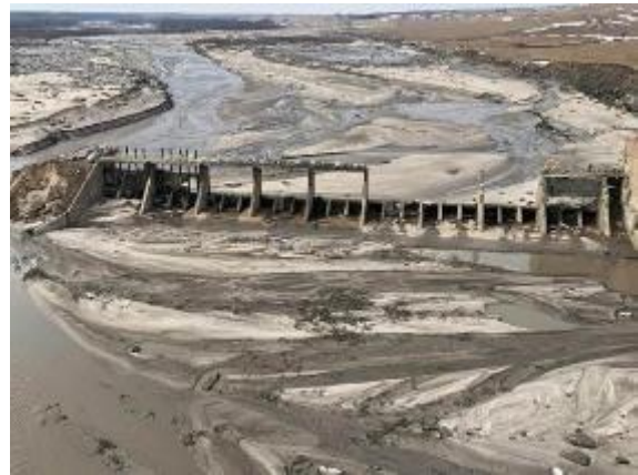
Figure B4- 2 The post-failure Spencer dam.
