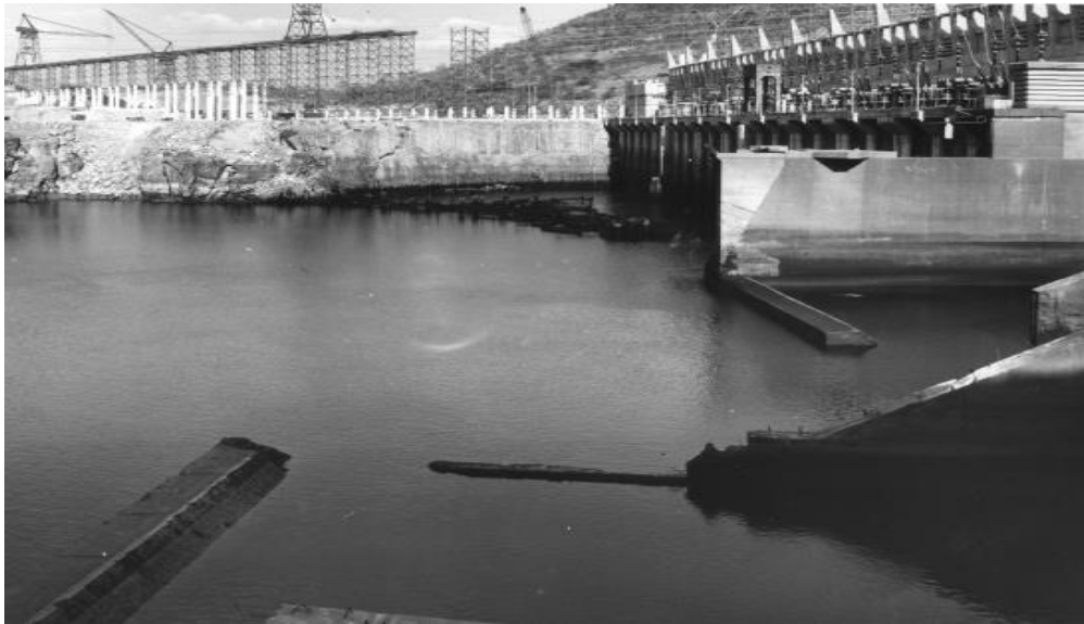
Figure B.1- 13 Photo taken where wall 3 is partially removed, and wall 2 is totally removed. In its terminal part, lip of flip bucket of Chute 2 is completely eroded. That situation precluded the placing of the floating bulkhead to initiate repairing works. (EDELCA)
