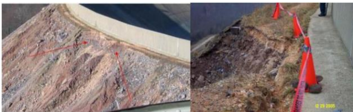
Figure B.2- 15 Erosion at Panels 48 and 49. Note scarps that may be the results of a localized slope failure. (FERC, 200&)
