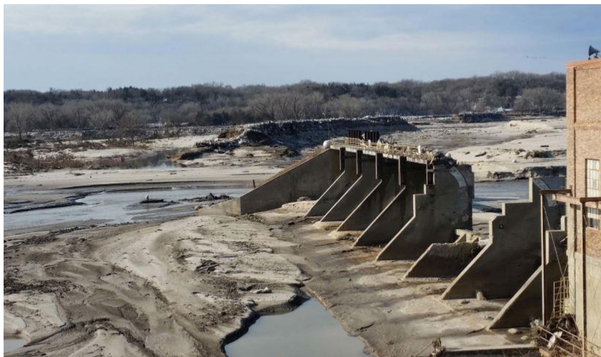
Spencer Dam after failure (Hydroreview.com, 2020)
