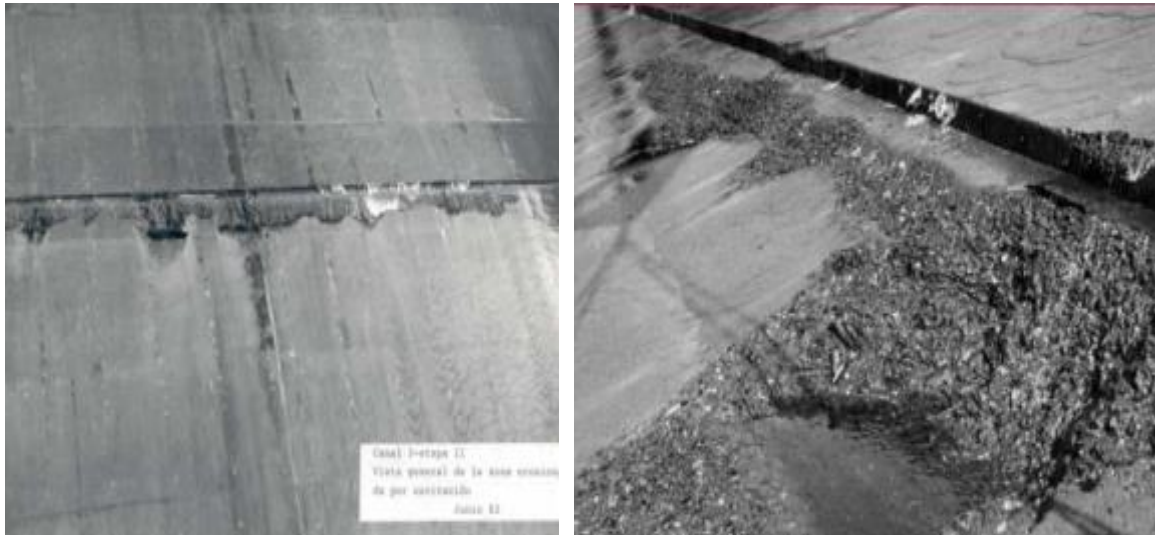
Figure B.1- 36 and Figure B.1- 37 Chute 3 Stage 2-Cavitation damage after 190 hours of operation with 2,000 m 3 /s (EDELCA)
