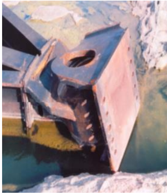
Figure B.6- 4 Spillway gate 5 tie beam left joint (weld joint not before failure to the designed penetration thickness). (CWC)
