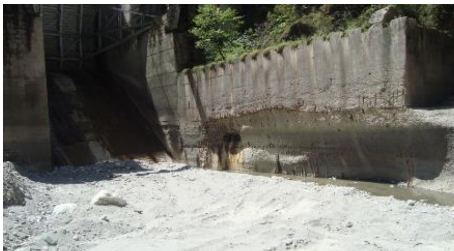
Figure B.5- 6 Damaged Left Training wall (CWC, 2017)
