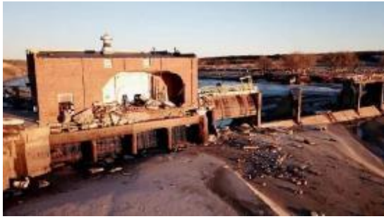
Figure B4- 8 Rain and snow melt take out Spencer Dam, 2019.
