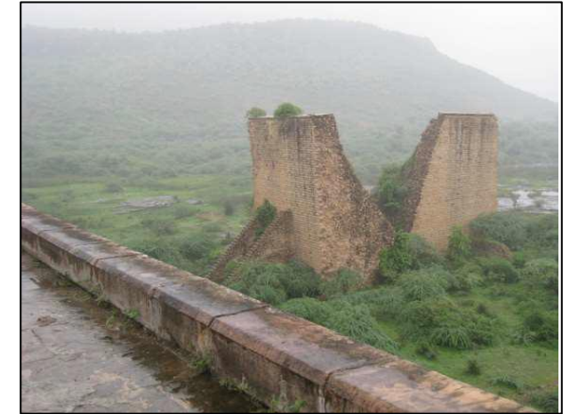
Tigra Dam failure
