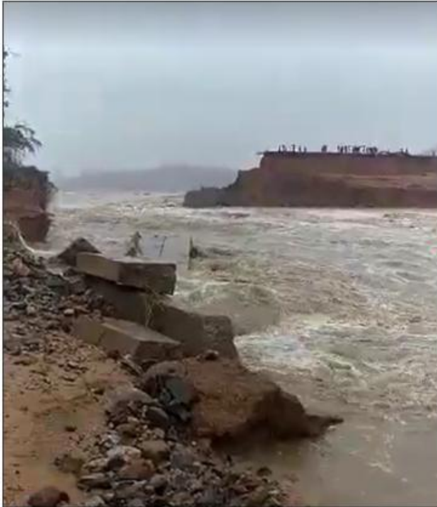
Pincha Dam Fails
